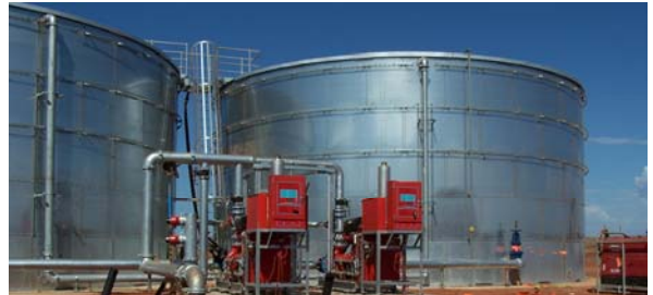
The West Kimberley Power Project
