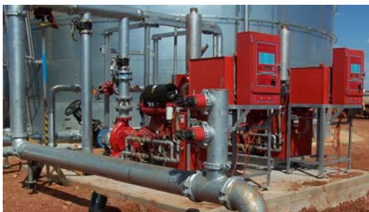
The West Kimberley Power Project
