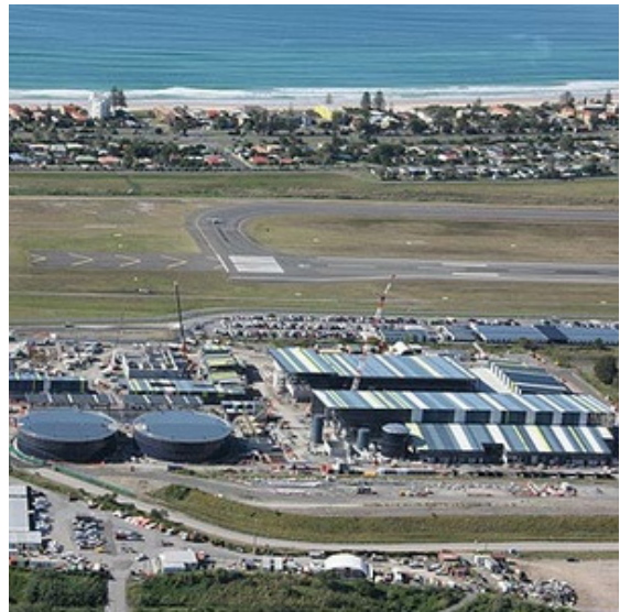
Aerial view of the Desalination plant
